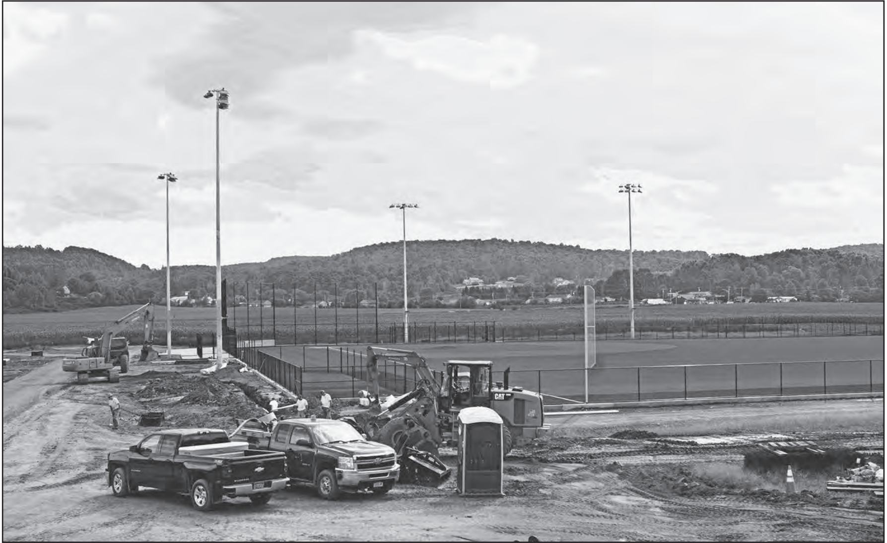
Work is done in October at the new Gutches Sports Complex Tuesday in Cortlandville.
